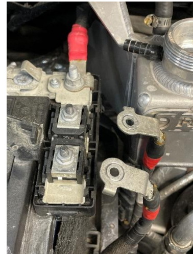
Figure 37: Reinstallation of each auxiliary cable to the positive terminal cluster.
