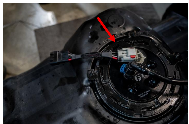
Figure 14: Installation of SureFlo sending unit, locking ring installed and highlighted with red arrow.
